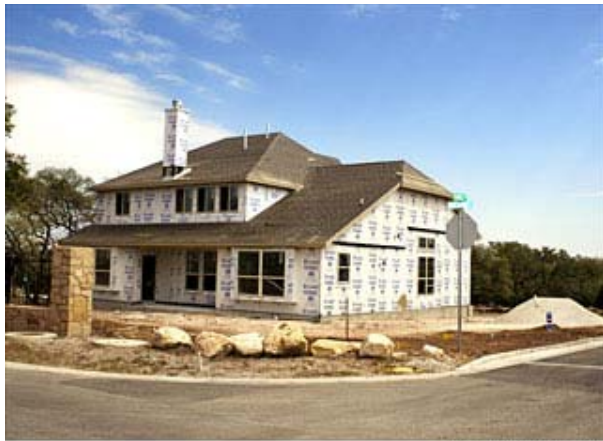
PHOTO: BRIAN FINKE A home under construction in Austin. The number of new homes in the pipeline nationwide is quite low.
